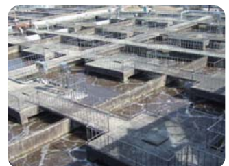
sewage treatment plantFreeco-Ex
